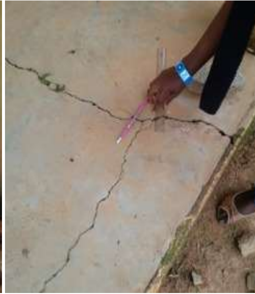
Figure 4: Cracks on floor
