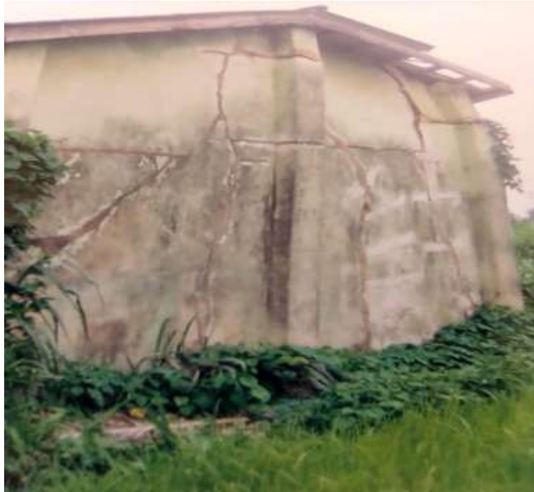
Fig. 7: Typical cracks caused by expansive soils on buildings at Bende, Southeastern Nigeria(adapted from Okoro et al. , 2019).
