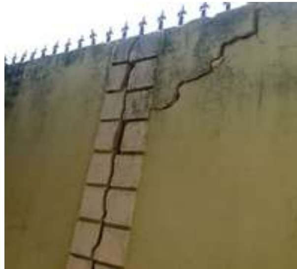
Figure 2: Vertical and diagonal cracks
